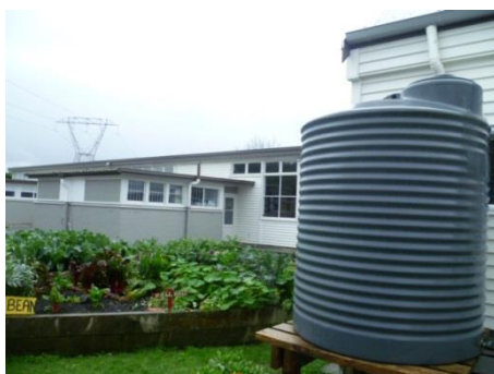
Water tank catching run-off from the school roof.
